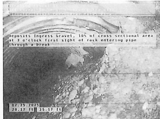
2, 00:00:00, 25.17ft Deposits Ingress Gravel, 10% of cross sectional area at 3 o'clock / first sight of rock entering pipe through a break North and South
