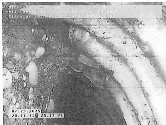
3, 00:00:00, 25.17ft Deposits Ingress Gravel, 10% of cross sectional area at 3 o'clock / first sight of rock entering pipe through a break North and South
