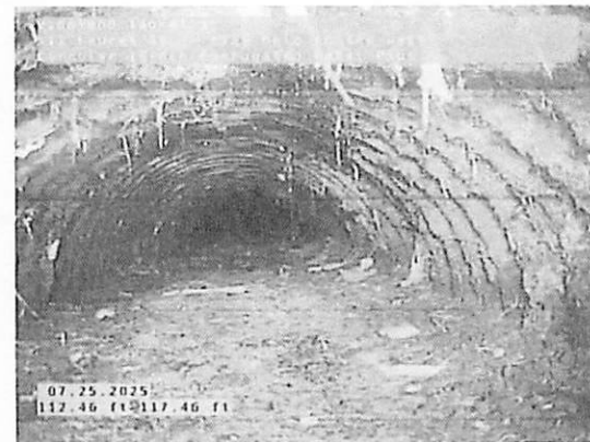
4, 00:00:00, 117.46ft General Observation / can not pass do to heavy debris sink hole is 128 ft camera stoped at 17
